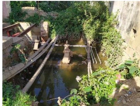
Leakages at the OHT
