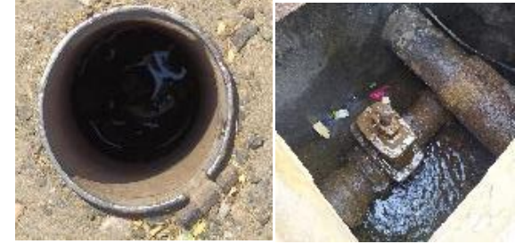
Leakages in valves in the Karelibaug command area
